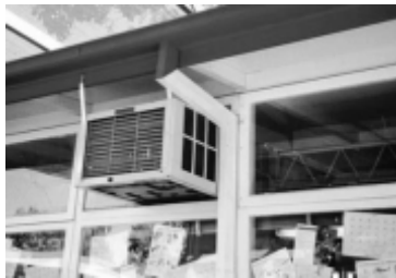
Window mounted air conditioning
