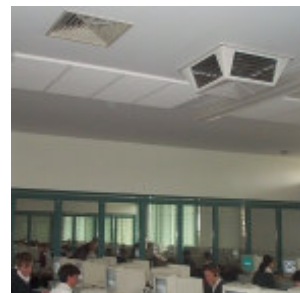
Evaporative cooling can be used in computer rooms
